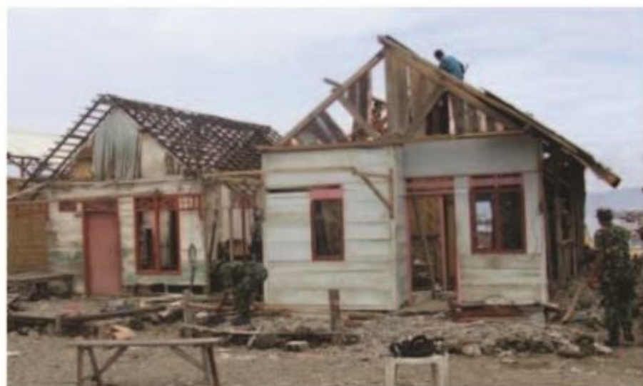
Upaya Penanganan Bencana Angin Topan di Kab. Tanggamus, Prov. Lampung. Sumber : BNPB Damages in the aftermath of the typhoon in Tanggamus, Lampung. Source: BNPB.
